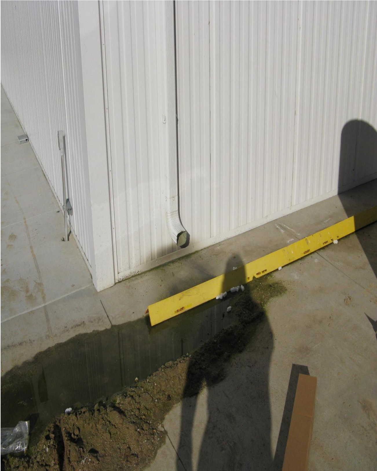
Figure 2c. Downspout from an adjacent warehouse
