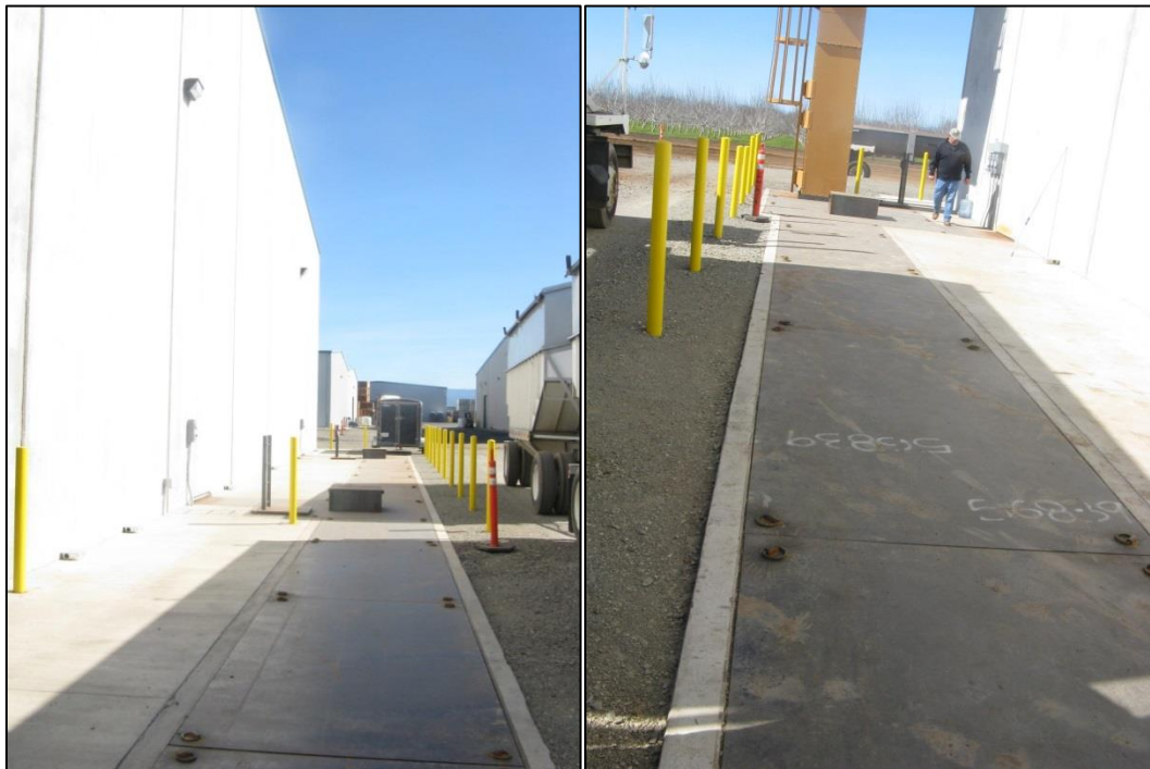
Figure Two: Steel plate conveyer trench covers
