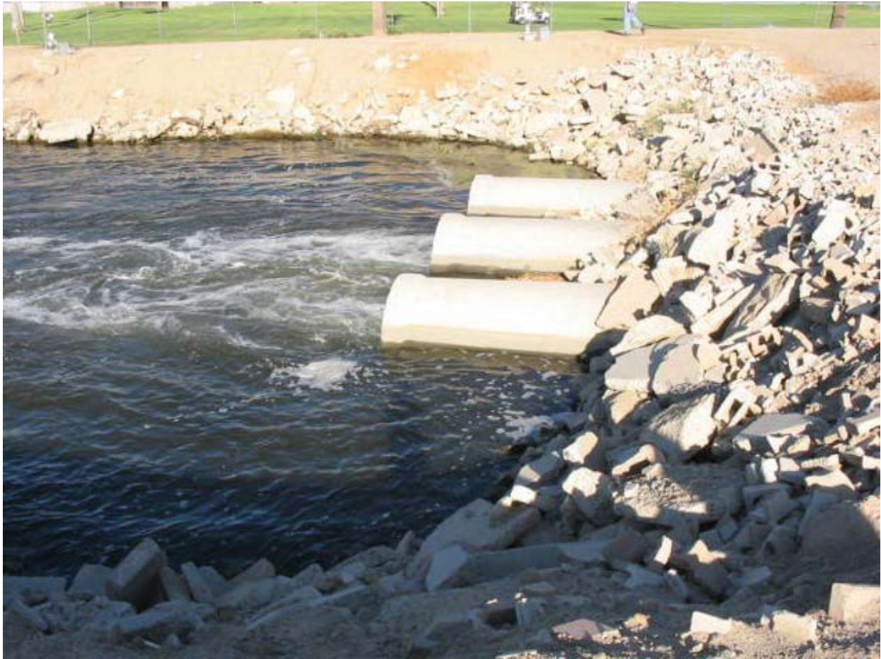
Middle pipe injected at upstream opening with Acrolein Head of Kern Island, Oildale, Kern County August 3, 2005
