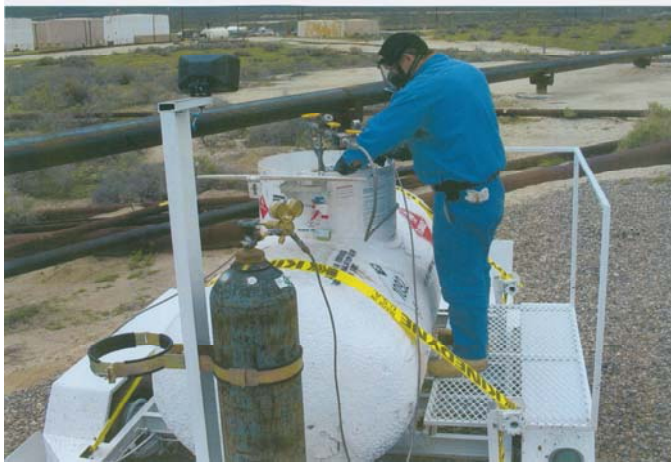
Photograph of an oilfield acrolein application showing a portion of a tank farm in the background. Courtesy of Baker Petrolite Corporation.
