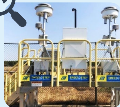
Monitoring station (9x9 ft)
