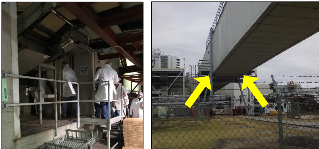
Figure 3. Walkway end on production-side of the facility (left). Exterior of walkway (right) with yellow arrows indicating the recommended location of the fans.
