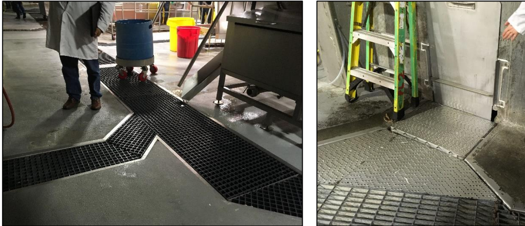
Figure 2. Floor gratings over drain system (left) provide a unique challenge to retaining the fumigant. One measure that could help is closing the door (right) to prevent gas movement out of the room.
